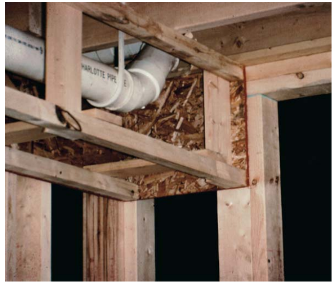
Photograph 9: Draftstopped Soffit —'Nuff said.
