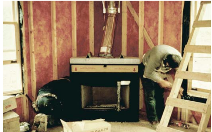
Photograph 3: Fireplace on Exterior Wall —OK, an even bigger hole than the bathtub hole. Kind of makes it funny to think about sealing an electrical wire going through a top plate when you have something this big.
