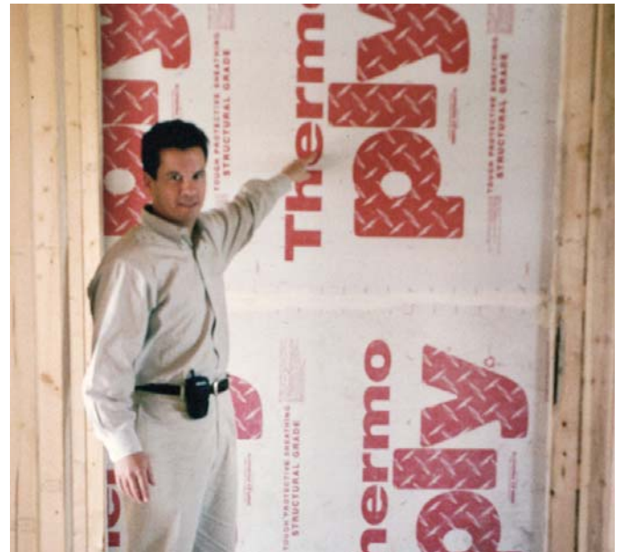
Photograph 6: Tub on Exterior Wall Before Tub Installation —Notice the rigid material on the exterior wall where the one-piece shower/tub thing is going to be.
