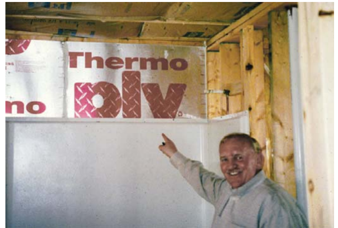
Photograph 7: Tub on Exterior Wall After Tub Installation —Notice the rigid material on the exterior wall behind where the one-piece shower/tub thing is. Notice the even bigger smile on that VP of construction.
