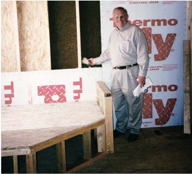
Photograph 5: Effective Draftstopping —Notice the rigid material behind the large soaking tub/whirlpool framing on the exterior wall. Notice the rigid material going up the exterior wall where the shower is going to be. Notice the big smile on the VP of construction for a major, major production home builder in Chicagoland. No comfort complaints for him anymore because there are no big holes.
