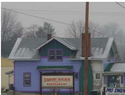
Snow melting because of bypasses in attic kneewall
