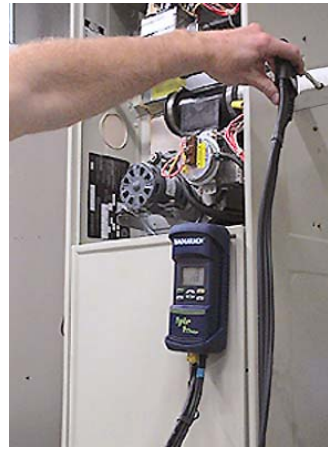
90+ Furnace: Measure draft and sample flue gases in the plastic vent pipe outside the furnace.
